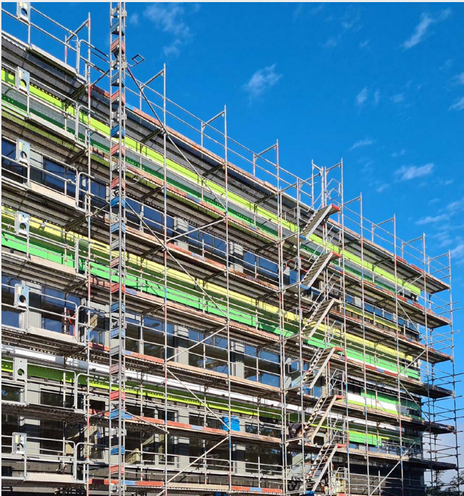
TITAN SLS heavy-duty props support the edges of the building during refurbishment of the facades
