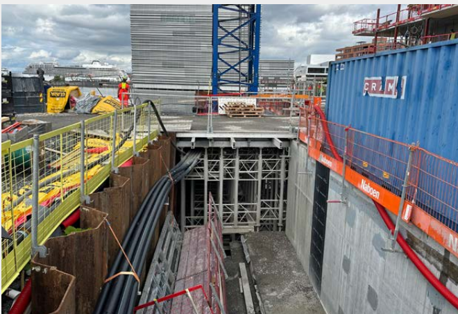
TITAN Megashore structure used as a bridge between the different construction phases
