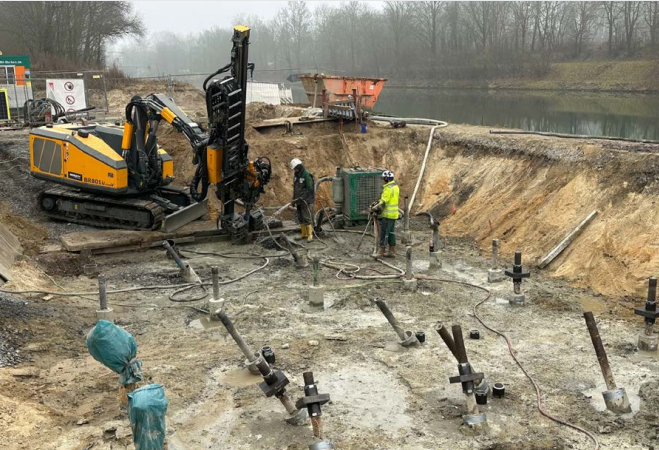
The micropiles were designed to be in a grid pattern which optimised the load distribution
