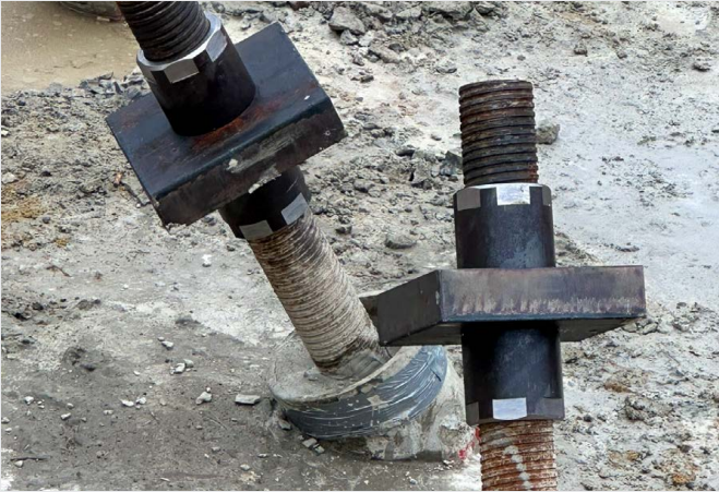
Vertical and inclined micropiles secure the abutment against compressive and horizontal forces.
