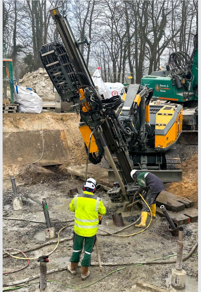
Installing a micropile with the TITAN self-drilling system; drilling and grouting are carried out in a single step
