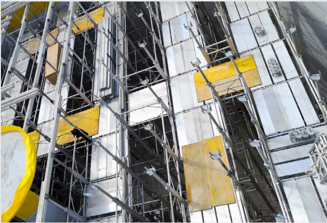
A secure assembly platform was erected at a height of around 10 m using aluminium scaffolding and decking planks
